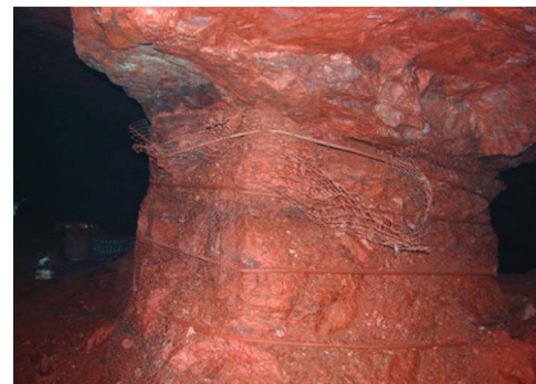
Figure 11—Example of reinforcement of a pillar using cables and mesh in the Santa Rosa mine. This is pillar f in Figure 10 (after Alejano et al. , 2017)
