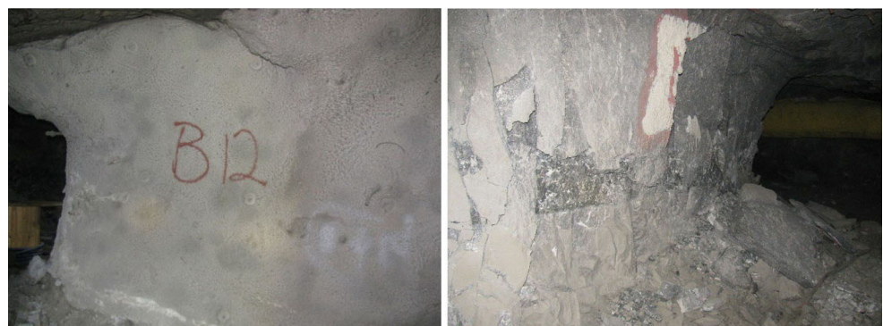
Figure 1—Application of a TSL stopped the Merensky pillar on the left from spalling. The pillar on the right was not reinforced and extensive spalling was observed
