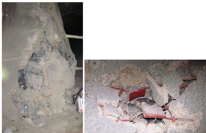
Figure 4—Failure of the pillar support illustrated in Figure 3. The photograph on the right illustrates the bolt pulling through the strap owing to the excessive dilation of the pillar (after Alejano et al. , 2017)
