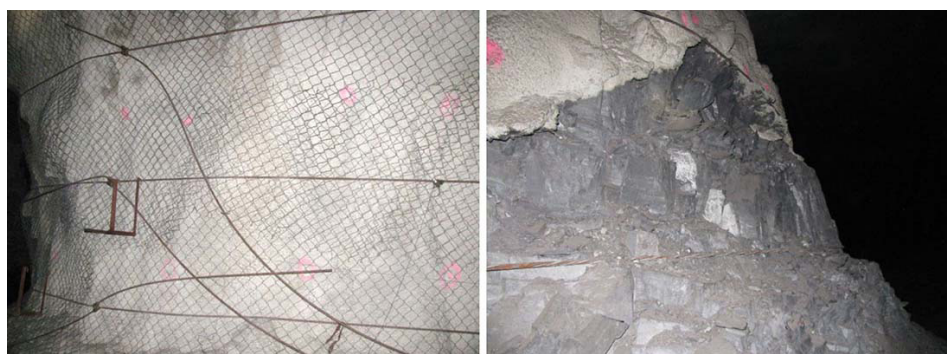
Figure 5—Support of a manganese pillar using TSL, mesh, and cable strapping. In some cases it works well (example on the left), but in other cases the liner could not stop the ongoing deterioration of a pillar (right)
