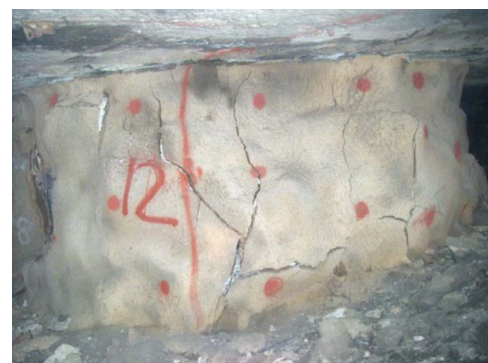
Figure 2—Ongoing failure of a pillar reinforced with shotcrete at the Everest mine (after Malan and Napier, 2011)
