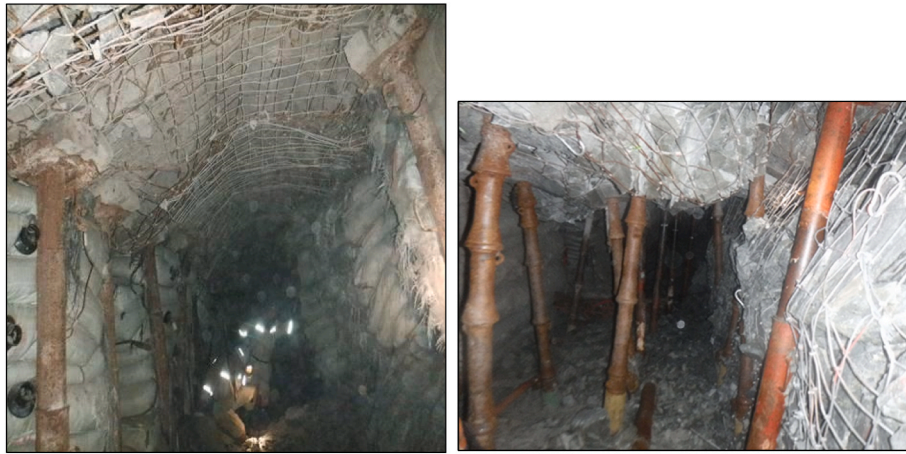
Fig. 6. Support used in the mining stopes in the Bamabanani shaft pillar. The face of the panel is shown the right (covered by the net). Note the extensive crushing of the face.
