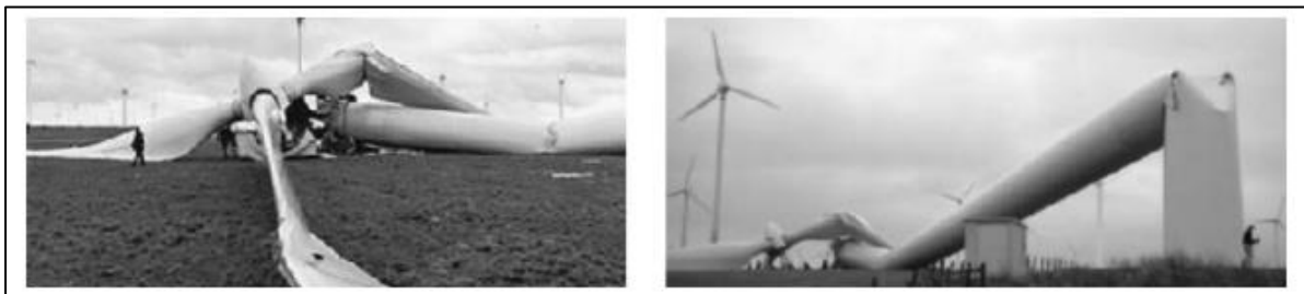
Figure 5: Total tower collapse (Ciang et al., 2008)
