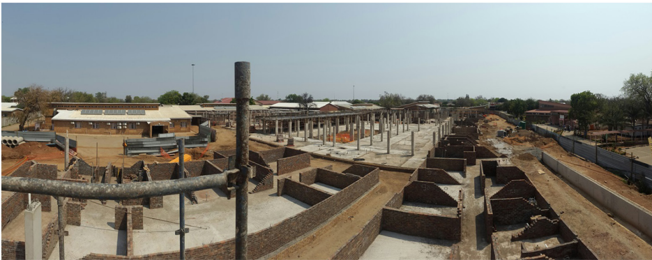
FIGURE 4 Construction of the new admissions, accident and emergency, radiology, pharmacy, and health support units at Maphutha Malatji Hospital (Roper, 2019).
