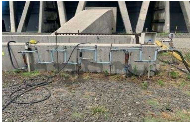
Figure S2 Overview of the coupon rack near the cooling tower basin.
