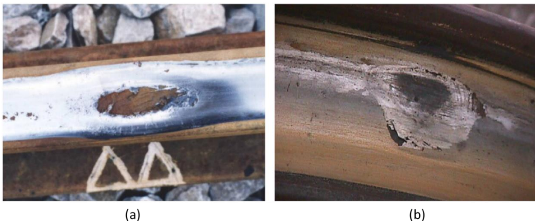
Figure 2.14: Example of wheel/rail damage in low adhesion conditions: (a) skidding marks on the rail surface and (b) wheel scratch on the tread [76].
