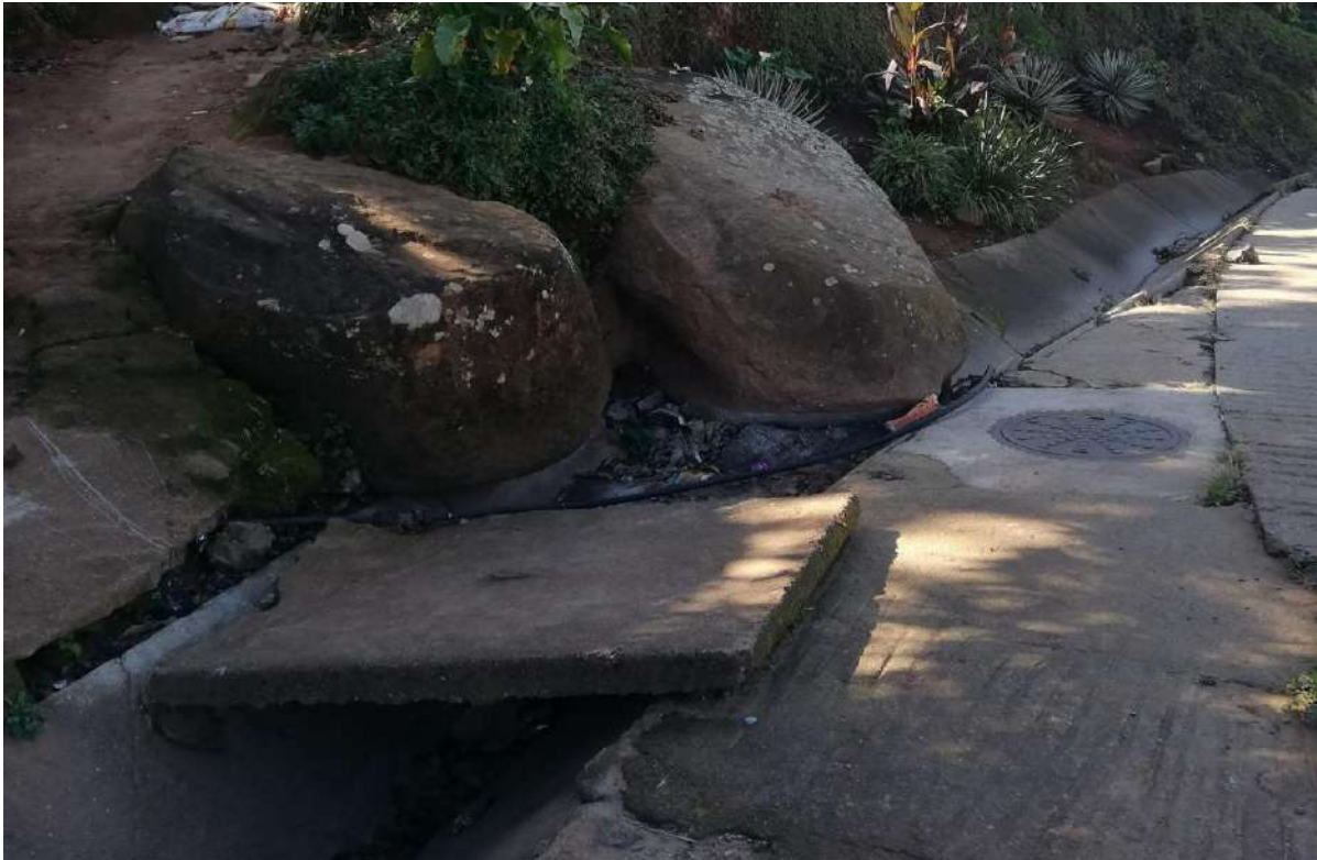
Figure 6.3. Blocked storm drains at Msunduzza
