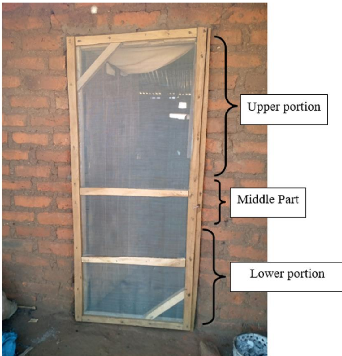
Fig. 2 A newly installed door screen showing the three portions considered in the questionnaire to assess damage
