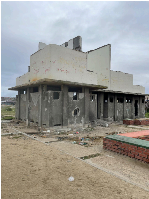
Figure 8: Damaged and vandalised VPPU building (Source: Author 2023)
