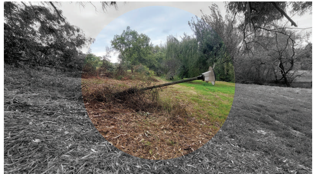
Damaged outdoor lighting network (Author, 2023)
