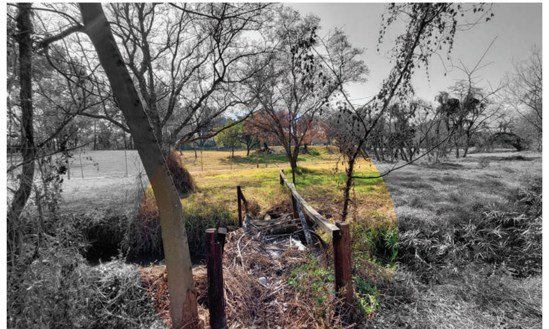
Dilapidated park bridges (Author, 2023)
