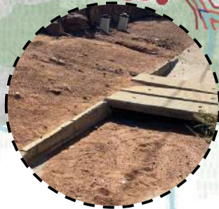
Drop Inlet Filled with sediment
