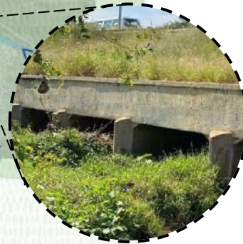
Box Culvert Overgrown vegetation, sedimentation, blocks water flow
