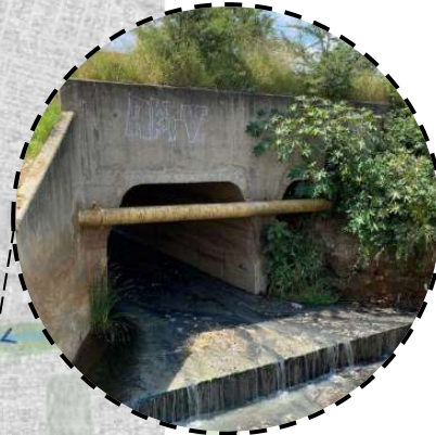
Box Culvert Carries pollution and sewage from Soshanguve Filled with sediment, blocking water flow
