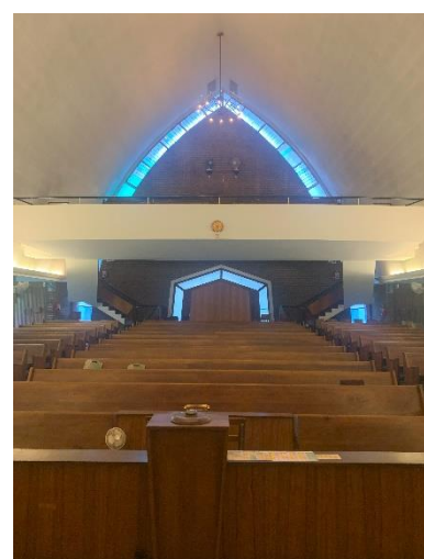
Figure 31: The rough plastered concrete balcony appears to be floating (Author, 2023).
