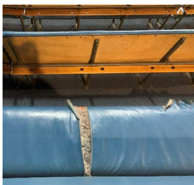
Figure 42: Lack of maintenance visible throughout (Author, 2023).
