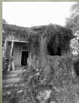
Fig. 8. Site Photo: Abandoned former houses, stripped by theft and no maintenance over a long period of time.
