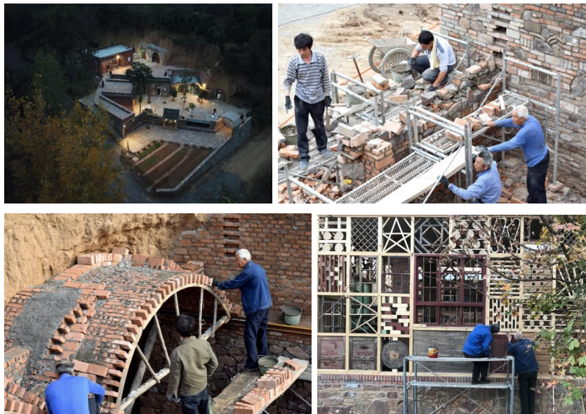
Figure 3.17 - House of Dreams construction photos, displaying masonry construction, reclaimed masonry walls and eclectic infill construction methods (Admin 2020).
