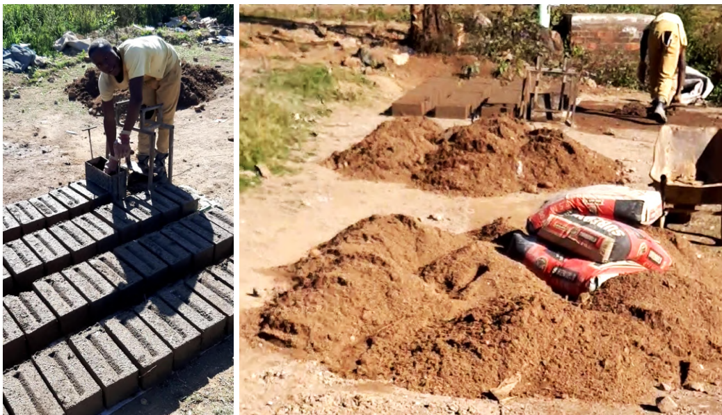
Figure.3.16 - A local entrepreneur making his own concrete blocks on the Open Green Space (Author 2022).
