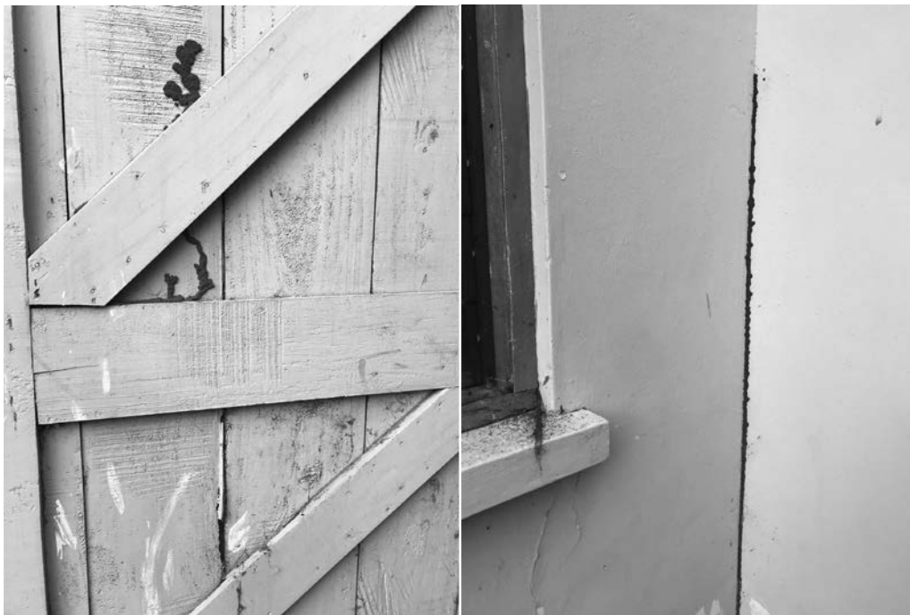
Fig. 3. Nsukka environmental challenge showing termite infestation in the location of the recorded materials.
