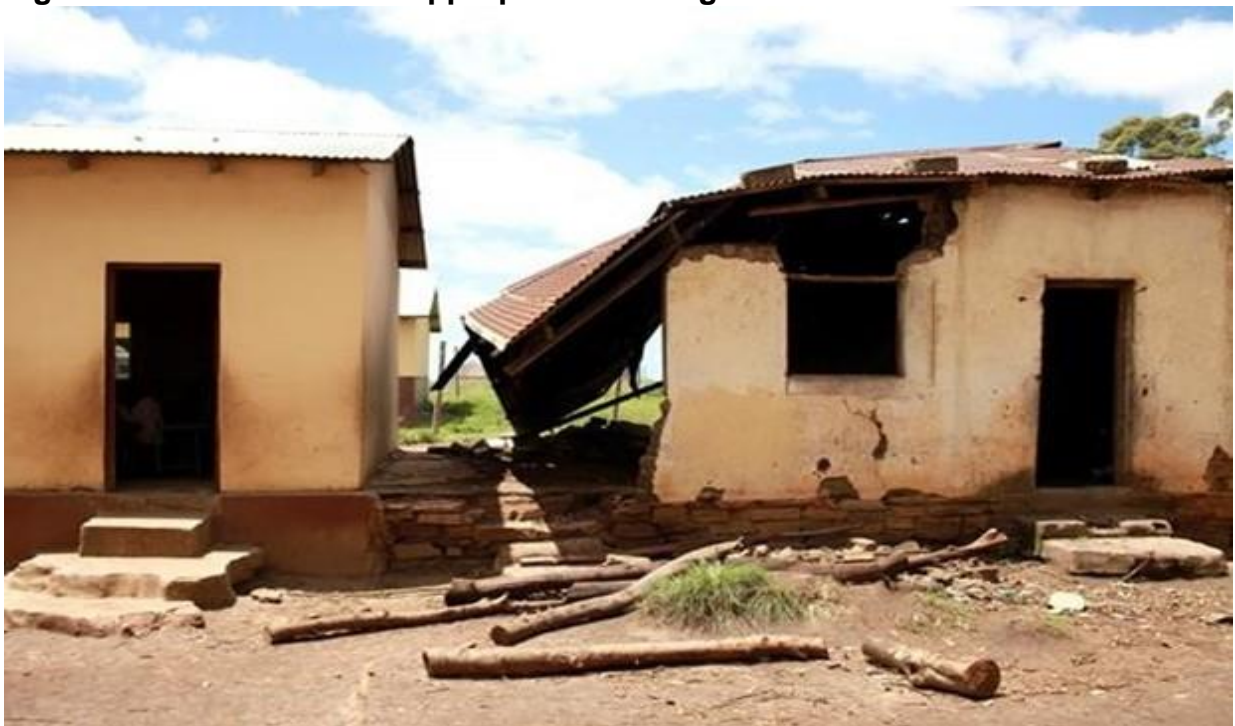
Figure 5.18: Evidence of inappropriate learning structures
