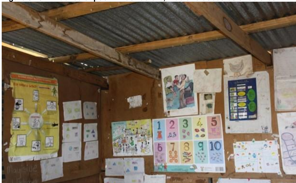
Figure 5.19: Evidence of poor infrastructure, mud and asbestos structures
