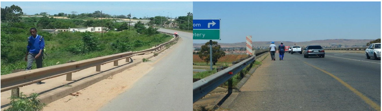
Figure 1: Defective guardrail installation - offering no protection to VRUs
