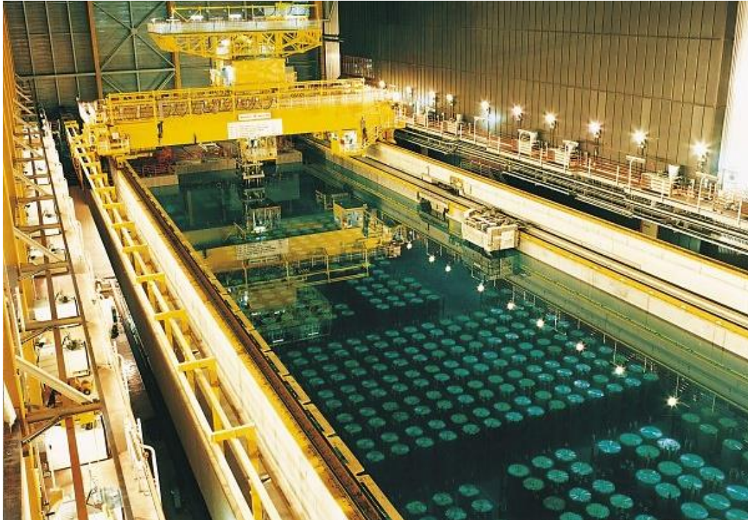
Figure 1.2. Storage pond for used fuel at the Thermal Oxide Reprocessing Plant (Thorp) at the UK's Sellafield site (Sellafield Ltd). Adapted from [www3].
