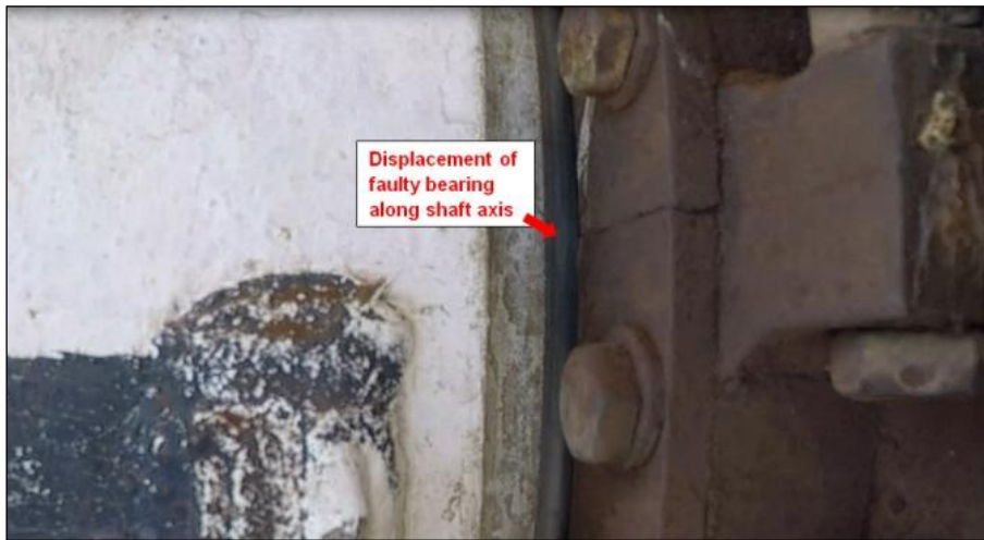
Figure 3.4 Bearing at west end of declination shaft shows displacement of \pm 10 mm. Photo credit: P. Mey.
