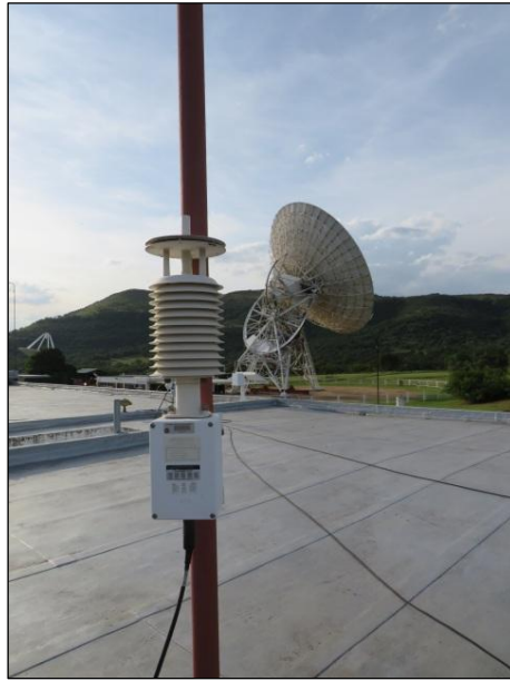
Figure 4.3 The Paroscientific MET3 unit of the HRAO IGS GNSS station used in the comparison is located on the roof of the facility's building. The new MET4 is temporarily installed ~12 m behind the MET3 (obscured by MET3 in image).
