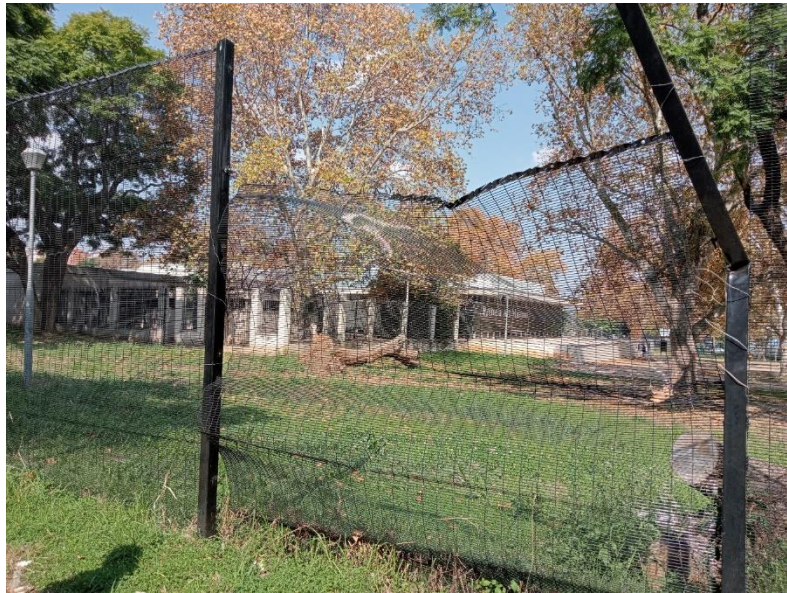
Fig 48: Fence areas that are broken aren't being repaired – this is about a years' time since it got damage (Author 2022).
