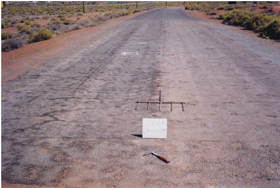
Figure 2: Condition after 20 years in February 1992 after brooming, showing left and right lanes of bitumen-rubber reseal in comparison with unresealed section in foreground, with an ASTM D4580-type chain drag
