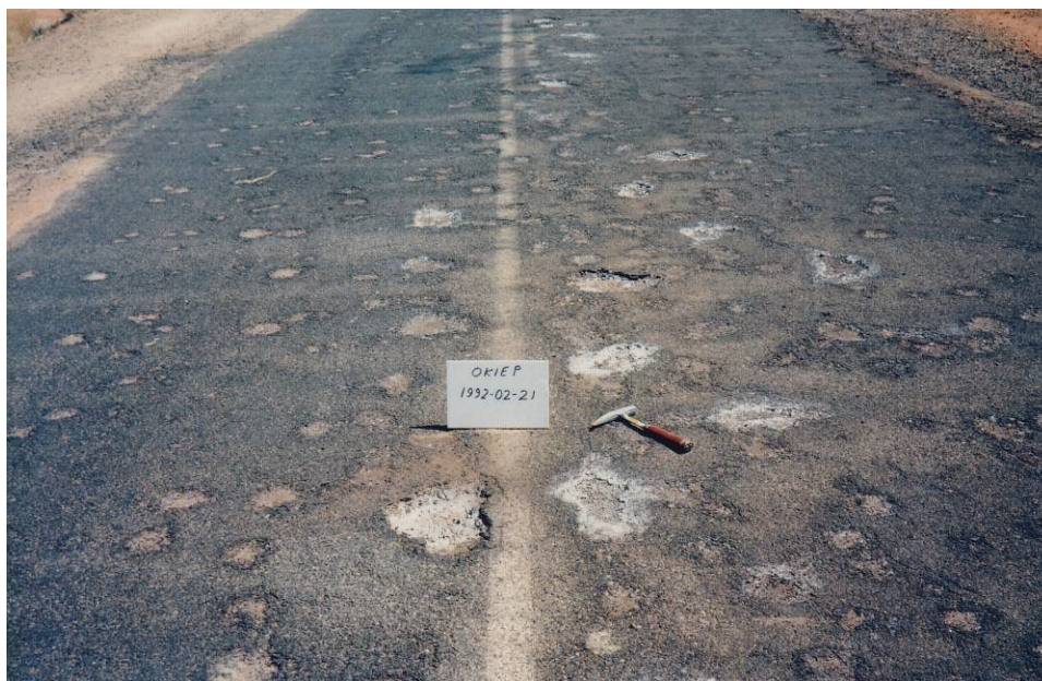
Figure 4: Light traffic and no maintenance caused the blisters to progress to white-stained craters and potholes
