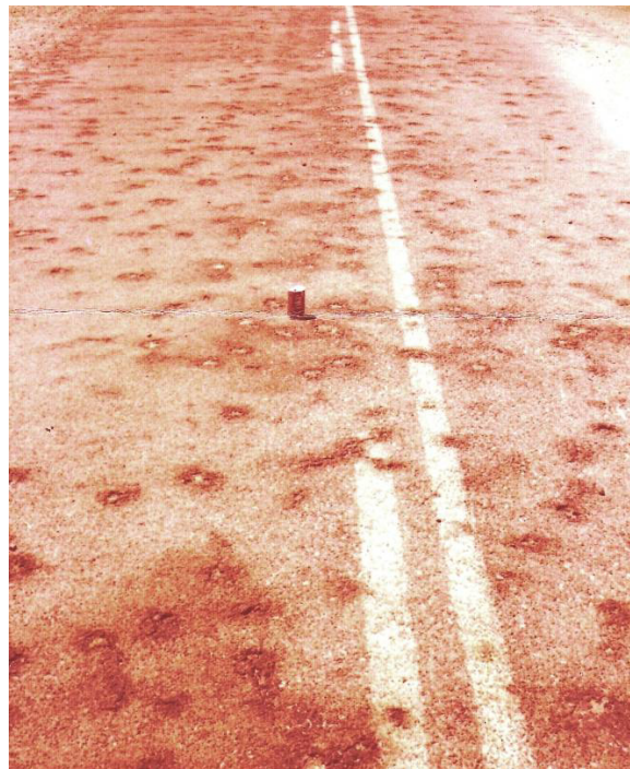
Figure 1: Condition in May 1984 showing damage under little traffic before spraying
