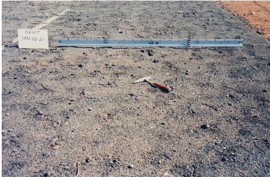
Figure 3: Lack of traffic led to blisters up to 30 mm high (but few potholes) on completely untrafficked section
