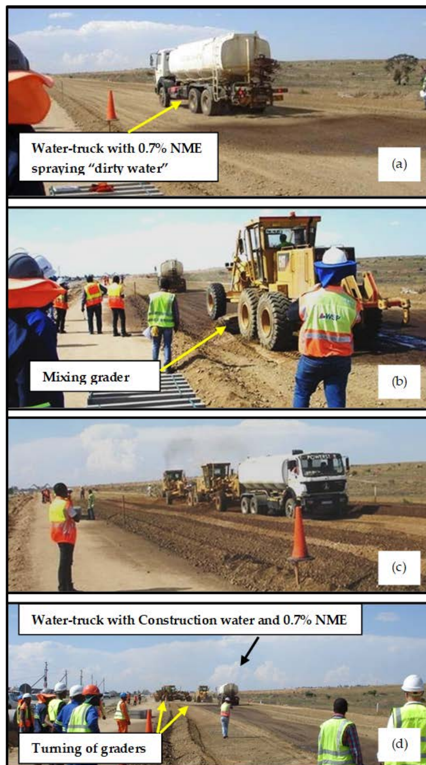
Figure 14. The granular material for the construction of the sub-base is spread along the section to be stabilised and compacted, allowing for the compaction factor. (a) The water-bowser containing the anionic NME pre-mixed with the required construction water is starting with the spraying of the NME mix. (b,c) The water-bowser is closely followed by graders that are mixing the NME stabilising agent with the construction water over the pre-determined length and width of the road. (d) Due to the turning movements and continued process of spraying and mixing, the construction of a section of road using conventional equipment is considerably more time consuming compared to the use of central mixing plants with paving equipment or with recycling equipment.
