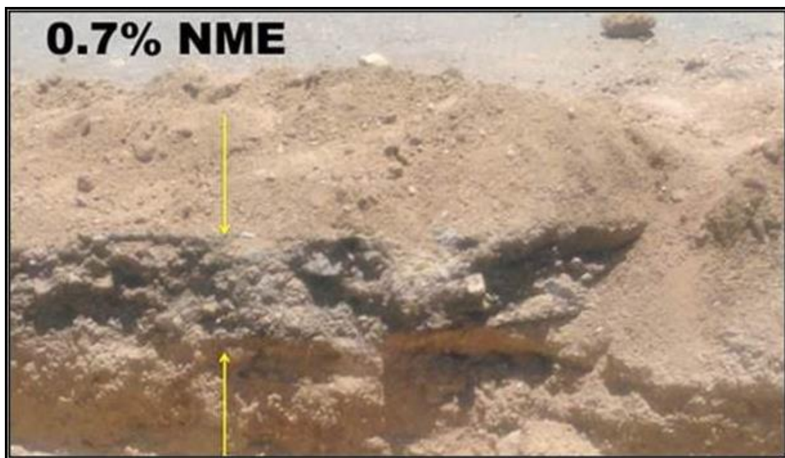
Figure 16. Cut through the stabilised sub-base constructed using a water-cart for distribution of the 0.7% anionic NME stabilising agent added to the construction water and mixed by grader, compacted as shown in Figures 14 and 15.
