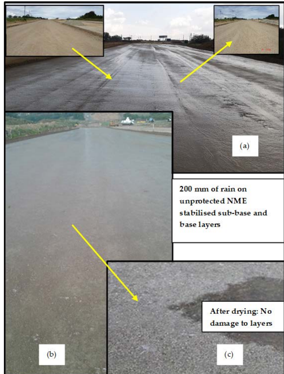
Figure 9. One week after placement of base (1.2% NME—0.7% residual bitumen) and the exposed sub-base (0.7% NME—0.4% residual bitumen), 200 mm of rain fell with (a) the sub-base-layer and (b) base-layer representing rivers. (c) After drying, no water-related damage could be observed.
