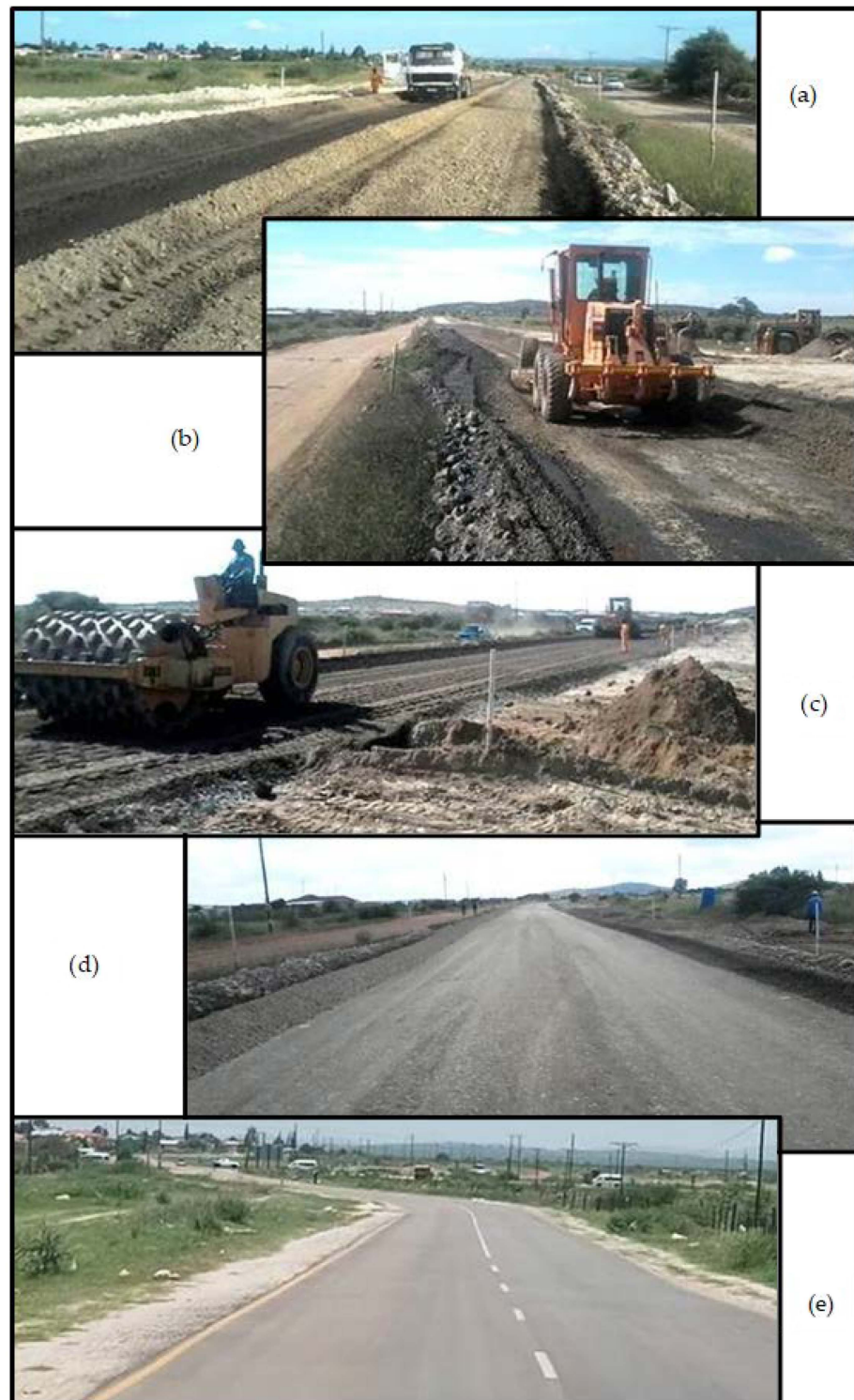
Figure 17. (a) Water-bowser with construction water and anionic NME stabilising agent. (b) Single grader used for mixing of the anionic NME stabilising agent pre-mixed within the construction water. (c) Compaction and cutting of final layer levels. (d) Condition of the compacted layer prior to applying a tack-coat and surfacing. (e) Condition of the surfaced road 6 years after completion.
