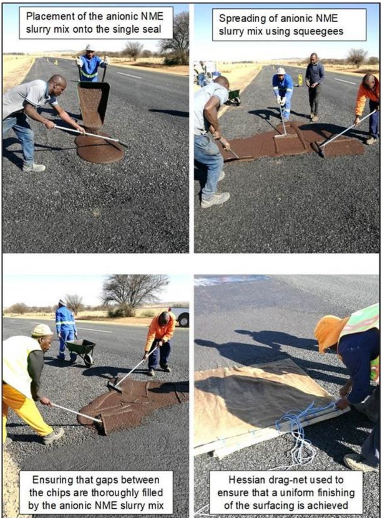
Figure 20. Labour-intensive construction of a modified cape seal using an anionic NME binder with the slurry mixed on site next to the road.
