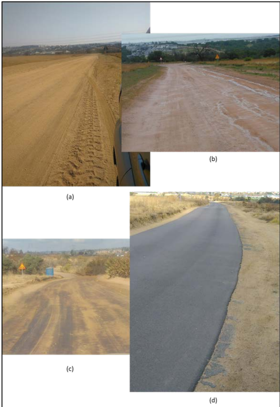
Figure 21. Upgrading of a local access road with (a,b) showing the sandy /slippery/muddy conditions prior to upgrading. (c) In total, 100 mm of in situ stabilisation with an anionic NME stabilising agent and (d) with an ultra-thin fine-graded asphalt surfacing (specified by client).
