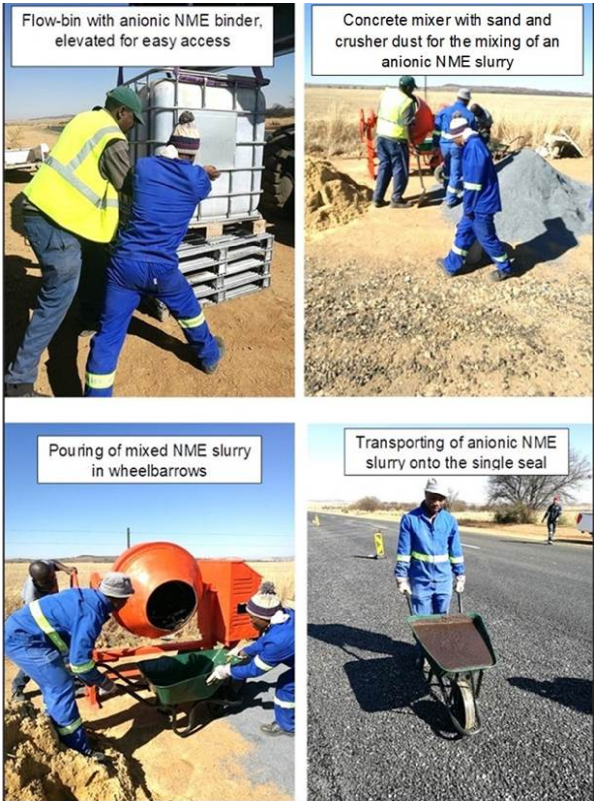
Figure 18. Labour-intensive road-side manufacturing of the slurry mix for a modified cape seal using an anionic NME binder.
