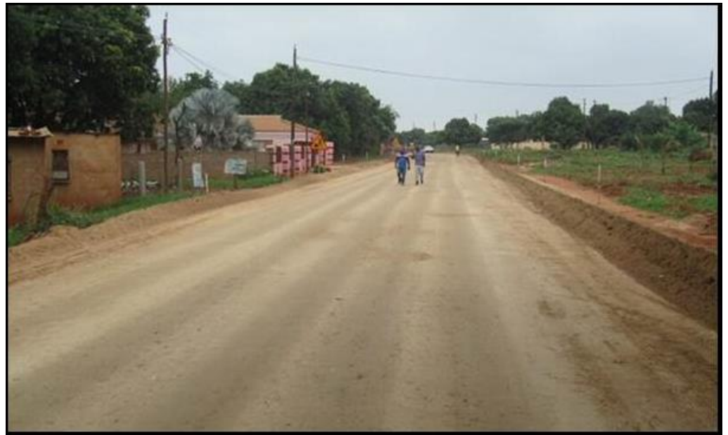
Figure 12. Recycled road with NME stabilisation opened to local traffic to provide access to houses, with no protective prime or surfacing added (note the same, pink-painted façade of the same house shown in Figure 11a).
