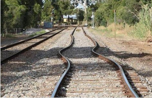
Figure 2.7: Rail kick out due to compressive forces
