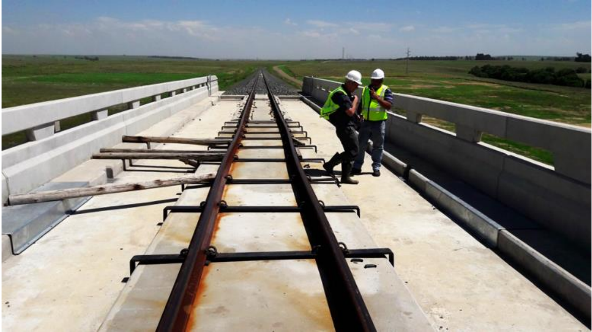
Figure 5.17: Lateral Buckling during Permanent Way Construction (prior to REJ installation)
