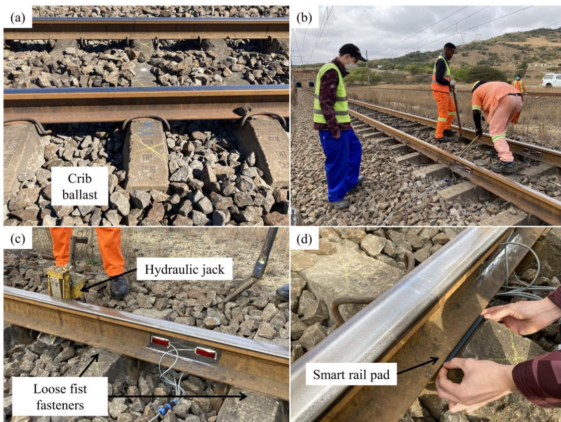
Figure 3.18: Rail pad replacement: (a) opening made for removing fist fasteners, (b) process of removing fist fasteners, (c) hydraulic jack to lift the rail and (d) the installation of the smart rail pad
