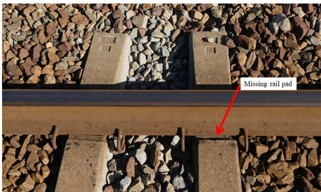
Figure 2.5: Ballast breakdown due to missing rail pad
