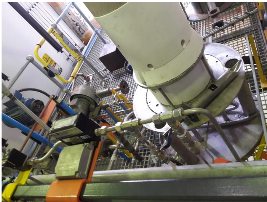
Figure 13: The inner refractory of the CRIPS 2 unit that separates the combustion and pyrolysis units. Note the two holes are for bed overflow and the skirting just below them
