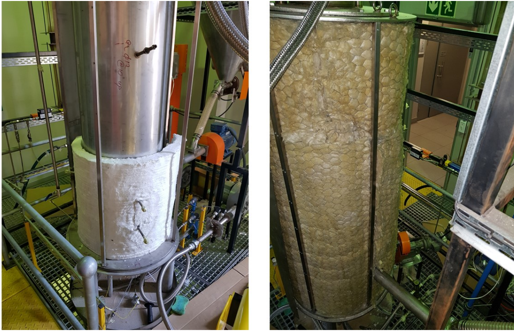
Figure 17: Insulation for the CRIPS 2 unit. Left: High-temperature inner insulation. Right: Reinforced outer insulation
