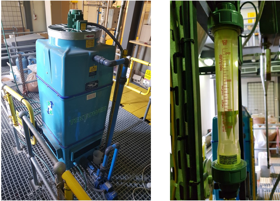
Figure 18: Left: Water cooling tower with delivery pump Right: Cooling water rotameter
