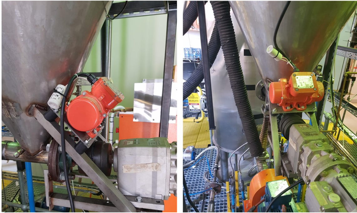
Figure 23: Side and rear view of the biomass hopper with the orange eccentric motor seated above the screw feeder coupling assembly
