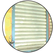
Roller Shutter Doors
