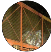
Steel Mesh Panel in Steel frame
