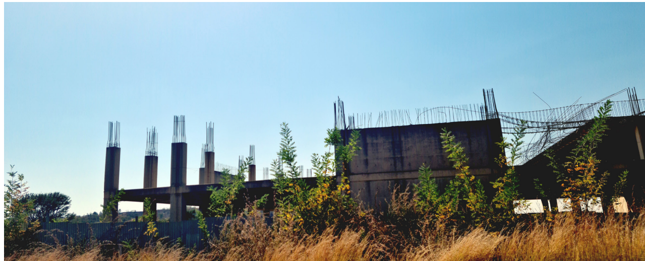
Figure.39: DE VILLA BOIS EXPOSED REBAR AND INCOMPLETE COLUMNS
