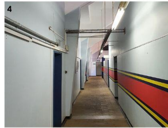
4 Long, narrow hallways in the swimming pool complex with no visual access to internal spaces.
