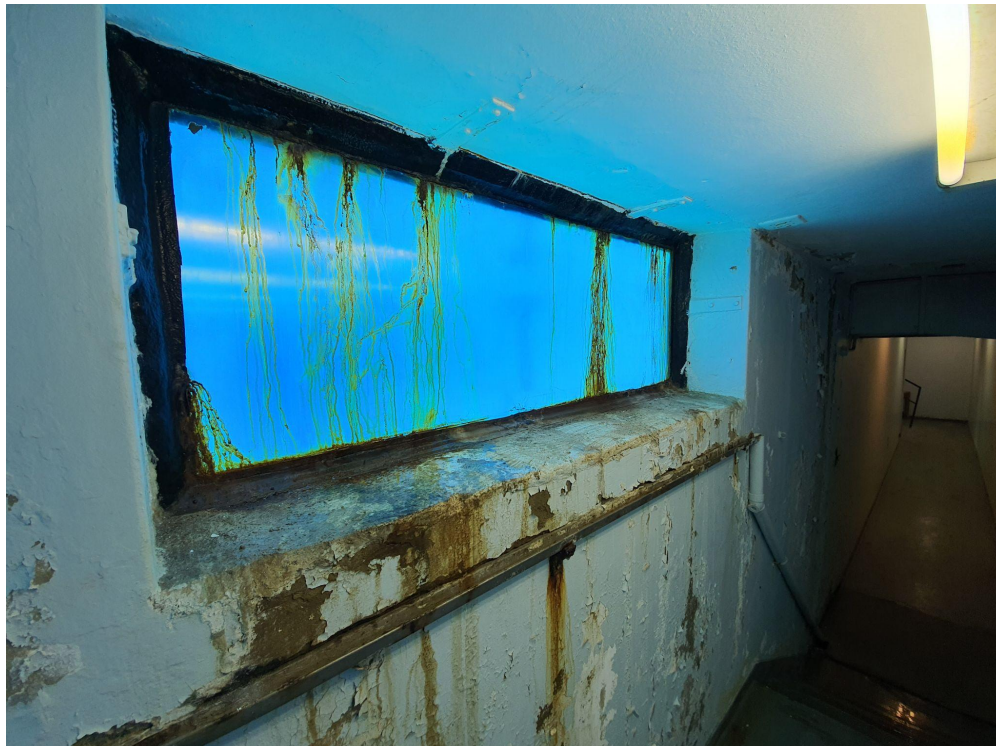
Figure 156: Waterproofing issues in the existing building (Author, 2021)
