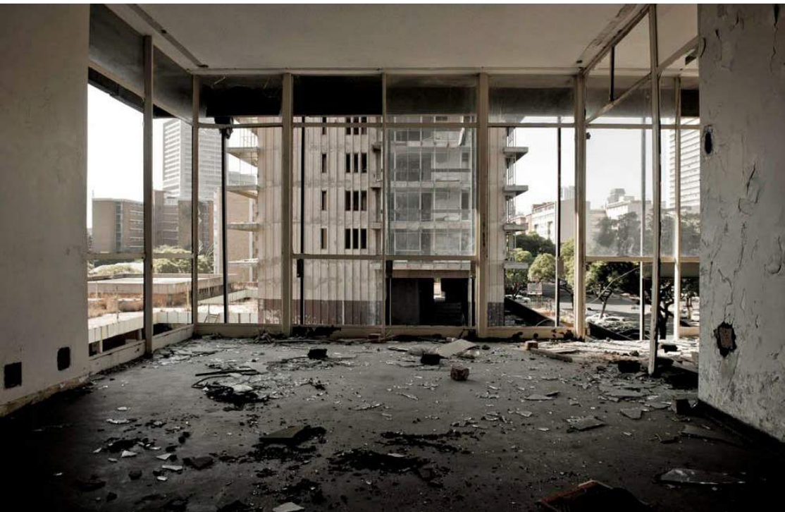
Fig.2: Schubart Park in a state of urban decay as it is found today (Verwey 2014).
