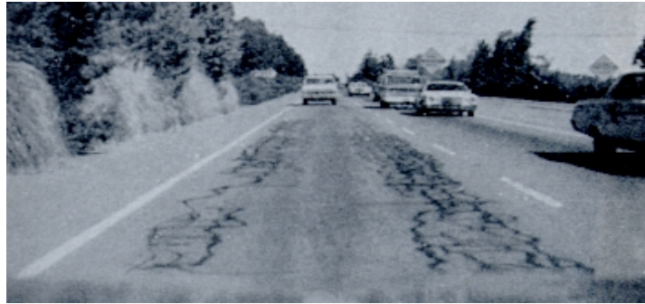
(b) Cracks in wheel tracks
