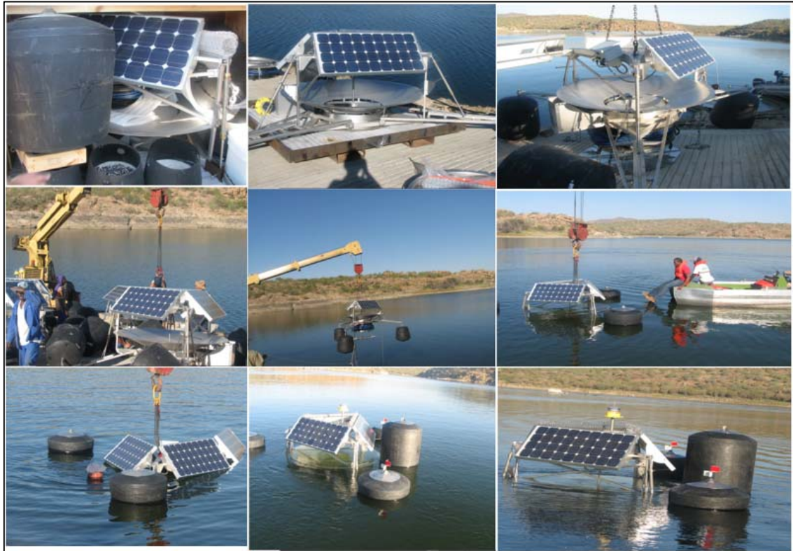
Figure 3: Pictures of Solar Powered Circulation installation as a phytoplankton control measure in the Swakoppoort Dam from 23 to 25 April 2013 for a period of 3 days.
