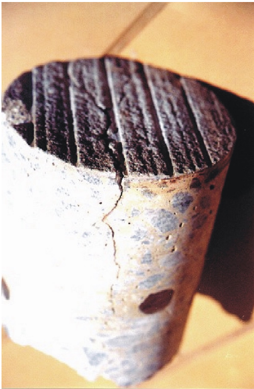
Photo 3: Intersection of transverse and random cracks with "pumping"
