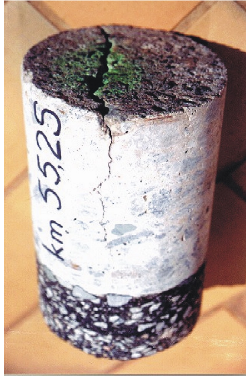
Photo 2: Transverse crack showing signs of "pumping"
