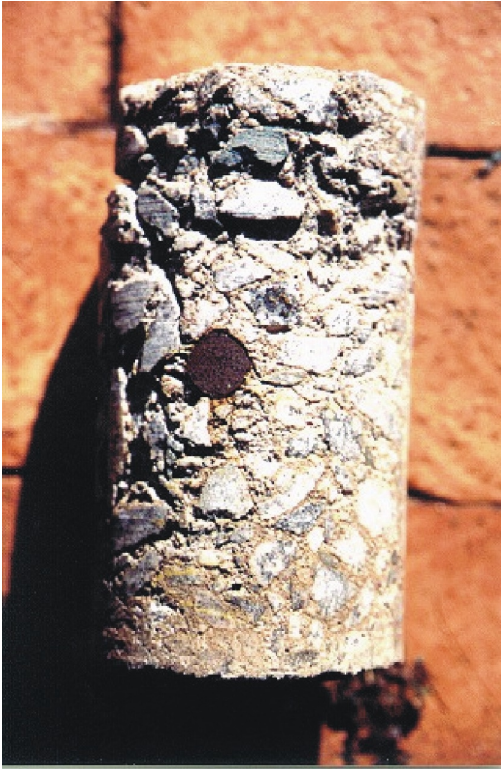
Photo 5: Weathering of concrete containing badly mixed cement/slagment mixture, after 10 years' exposure to elements
