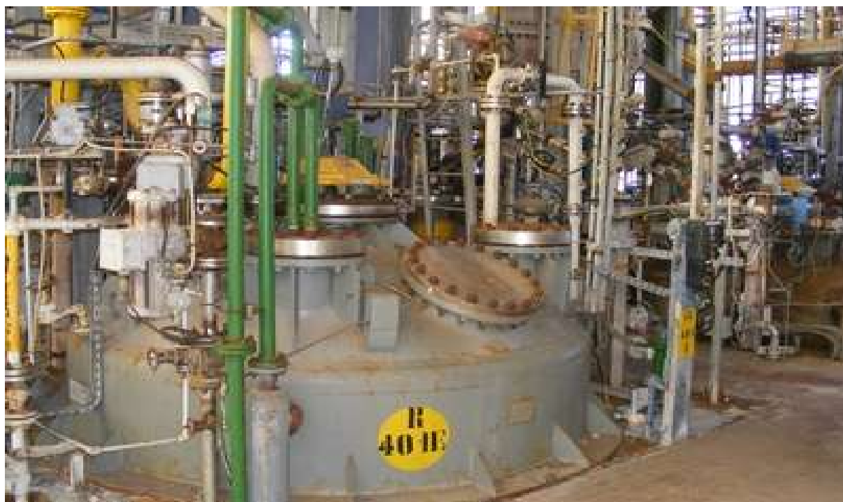
Figure 5: Head section of an industrial 40-kL polymerisation reactor (Images courtesy of International Process Plants).
