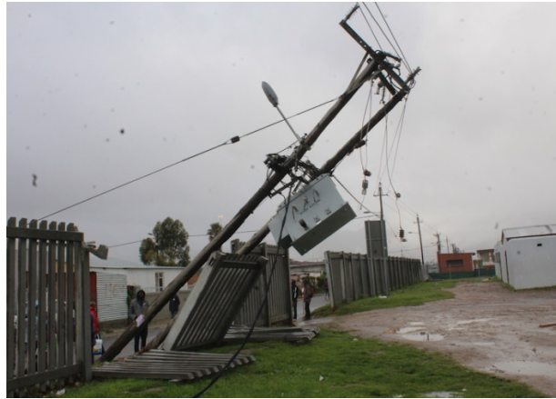
Figure 20: An electricity pole blown over in Nomzamo, 7 June 2017.
