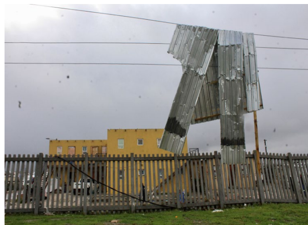
Figure 22: The roof blown off house in Nomzamo.
