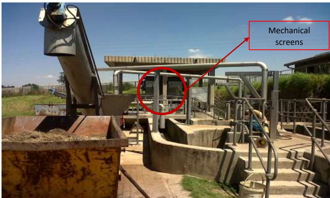
Figure 9: Naauwpoort WWTP Inlet works
