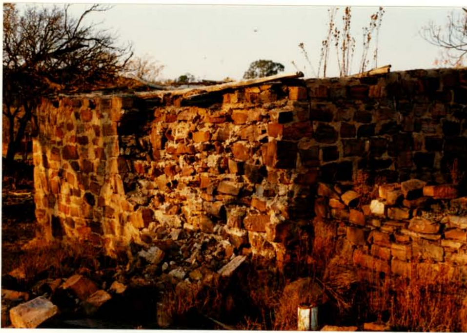
WEST VIEW OF 11.26 SHOWING SPLIT WALL & WOODEN ROOF BEAMS
