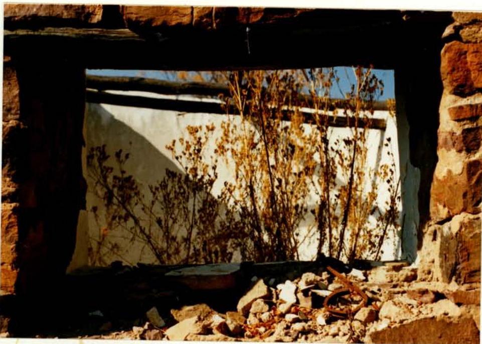
DETAIL OF WOODEN LINTEL OF 11.26 ABOVE WINDOW (from outside) NOTE THE ROOF BEAMS IN THE BACKGROUND
