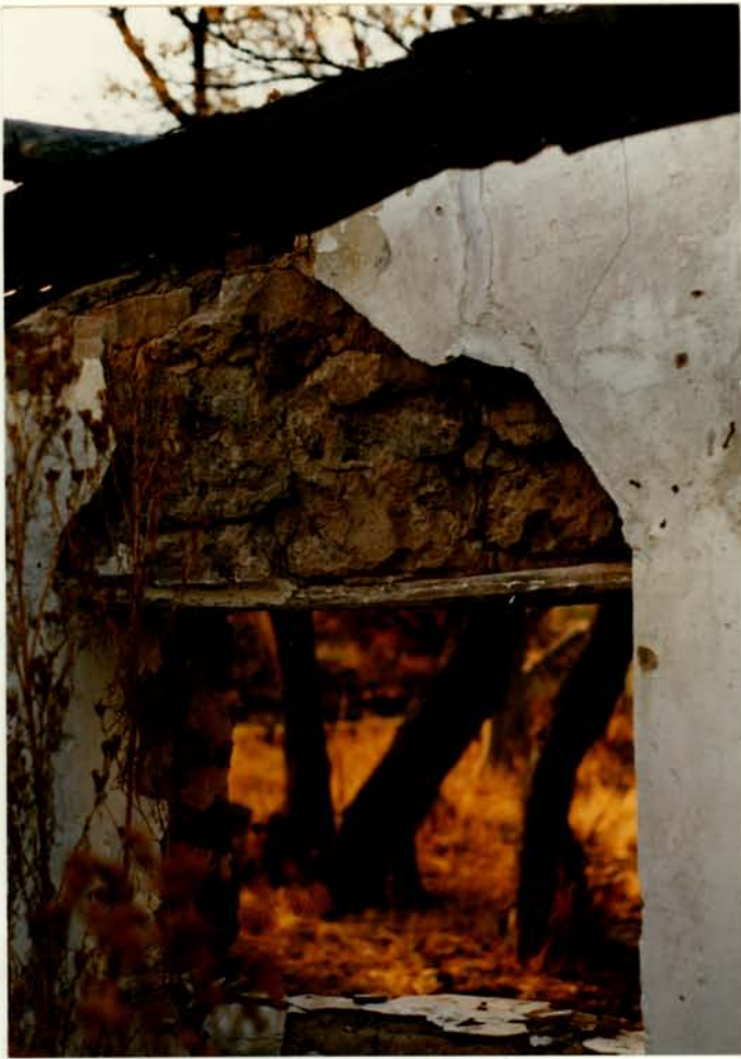
inside view of the window in 11.20 NOTE THE INSIDE PLASTER
