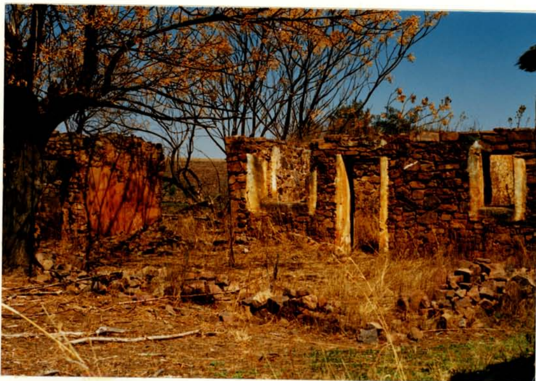
BUILDINGS 71.23 & 11.24 . PROBABLY EARLY DWELLINGS 4 NOTE THE BAD CONDITION OF THE GARDEN WALL
