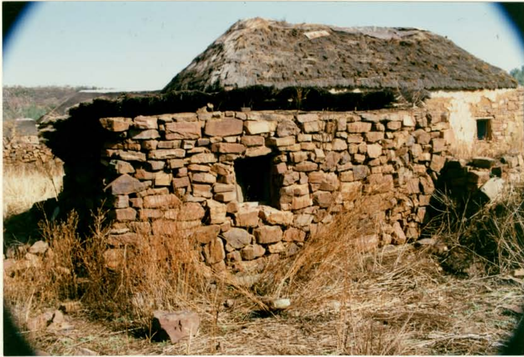
PHOTO 1.3. EAST ELEVATION OF BUILDING 11.13 WITH COLLAPSED ROOF
