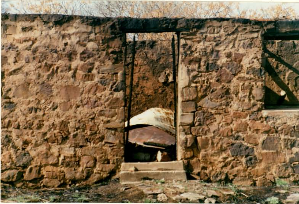
4. DOOR FRAME ON NORTH ELEVATION OF BUILDING 11.2.
