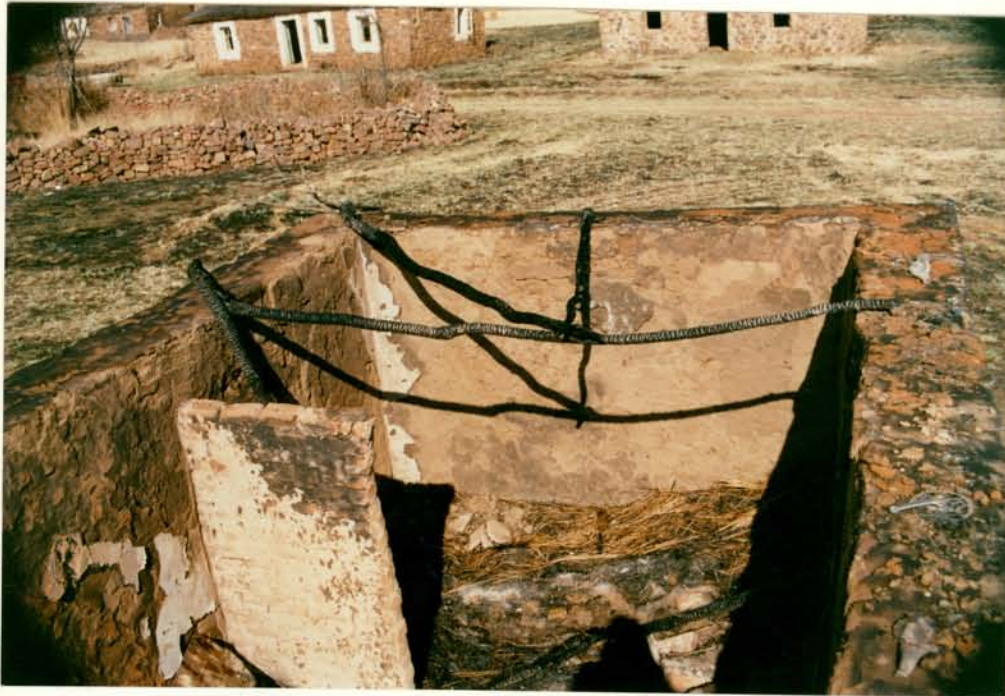
5. BURNT TRUSS ON WEST SIDE OF BUILDING 11.2.
