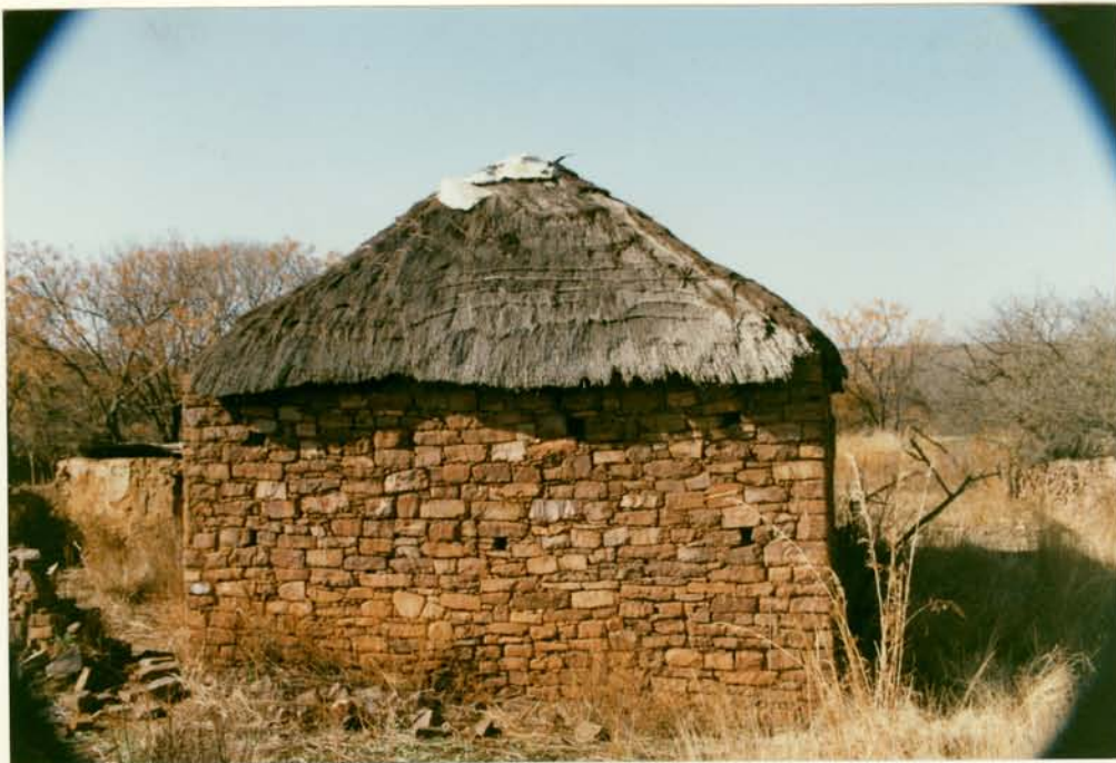
2. NORTH ELEVATION OF BUILDING 11.12 WITH HOLES IN THE WALL
