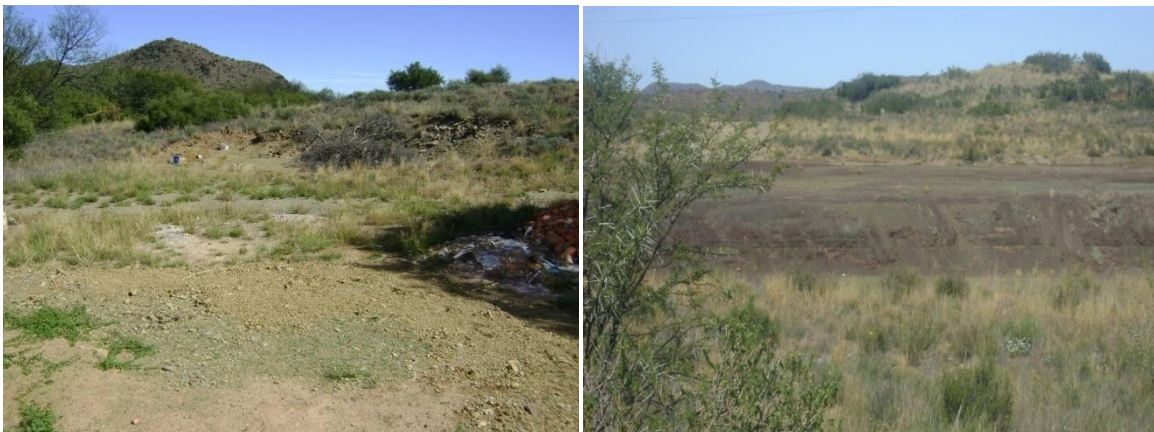
Figure 11 a. Building rubble lying on site, b. lack of rehabilitation with high soil erosion potential
