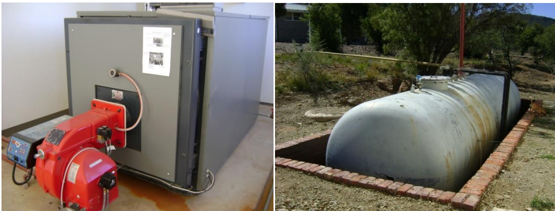
Figure 7 a. hot water boiler body, b. 30 000l diesel tank, feeding into the boiler (Fraser, 2013)
