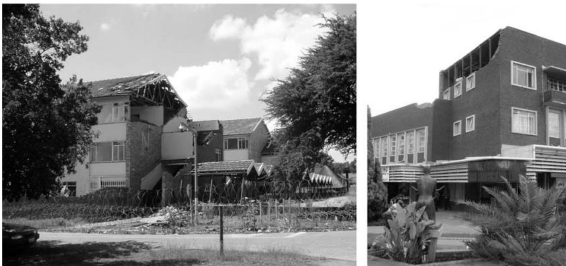
Figure 2-9 Structural damage due to the Stilfontein tremor of ML = 5.3 on 9 March 2005 (Linzer et al., 2007)
