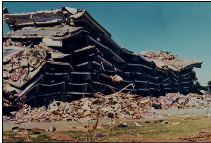
Figure 2-6 Collapse of a six-storey high block of flats due to the 1976 Welkom seismic event (Kijko et.al, 2015)
