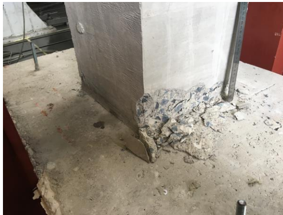
Figure 4-31 Crushing of the concrete during the 1 g experiment
