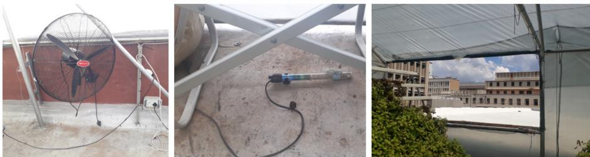
Figure 89: Measures taken to improve the indoor environment. Photos taken at Stanop building and Minerals Council farms.
