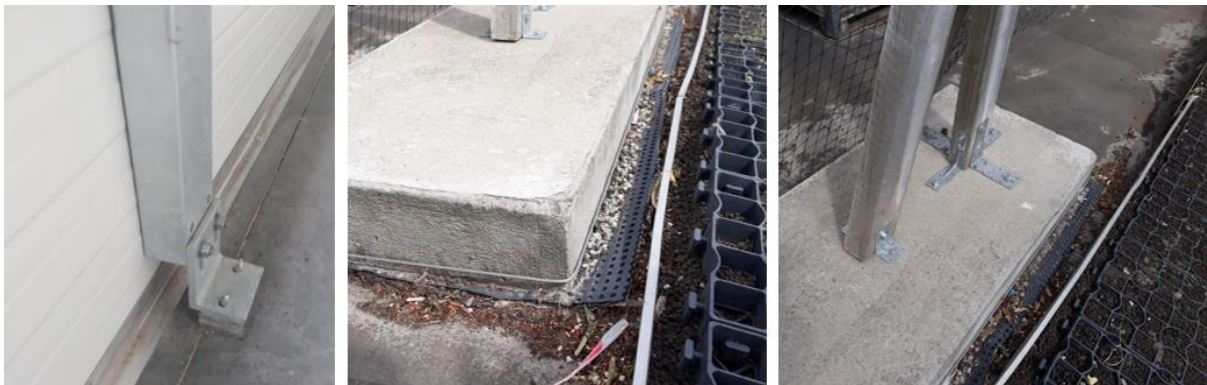
Figure 52: Layered fixing of farm structures and equipment to minimise damage to the existing structures. Location: Belgium.
