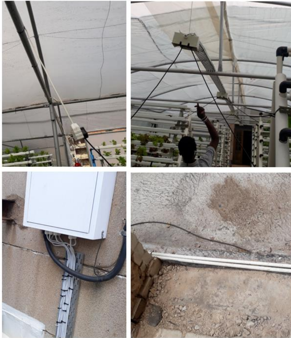
Figure 46: Reticulation of electricity throughout a typical South African rooftop greenhouse (BIA). Location: South Africa.
