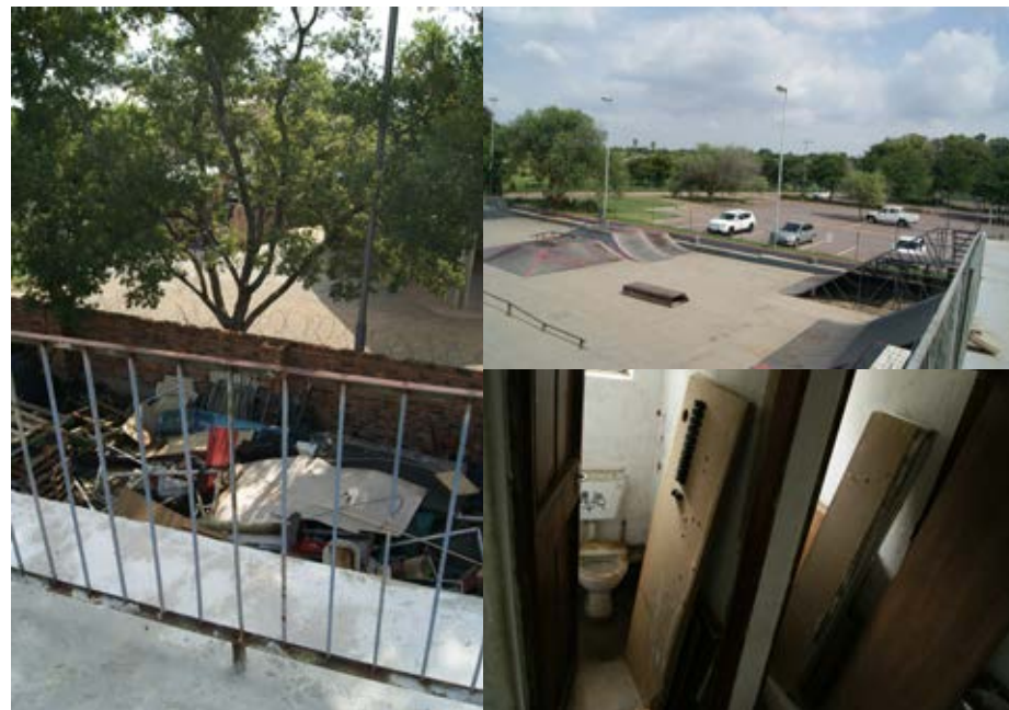
FIGURE 52. Degradation on site and plumbing issues (Author, 2020)
