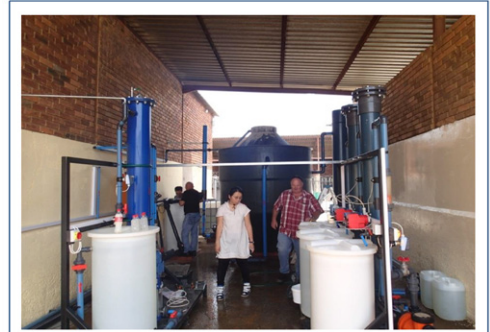
Complete DAF Unit
