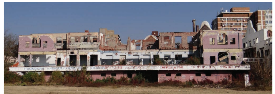
Figure 4.8. Current Damaged state of Southern Clubhouse (Bruwer & Paine 2017)
