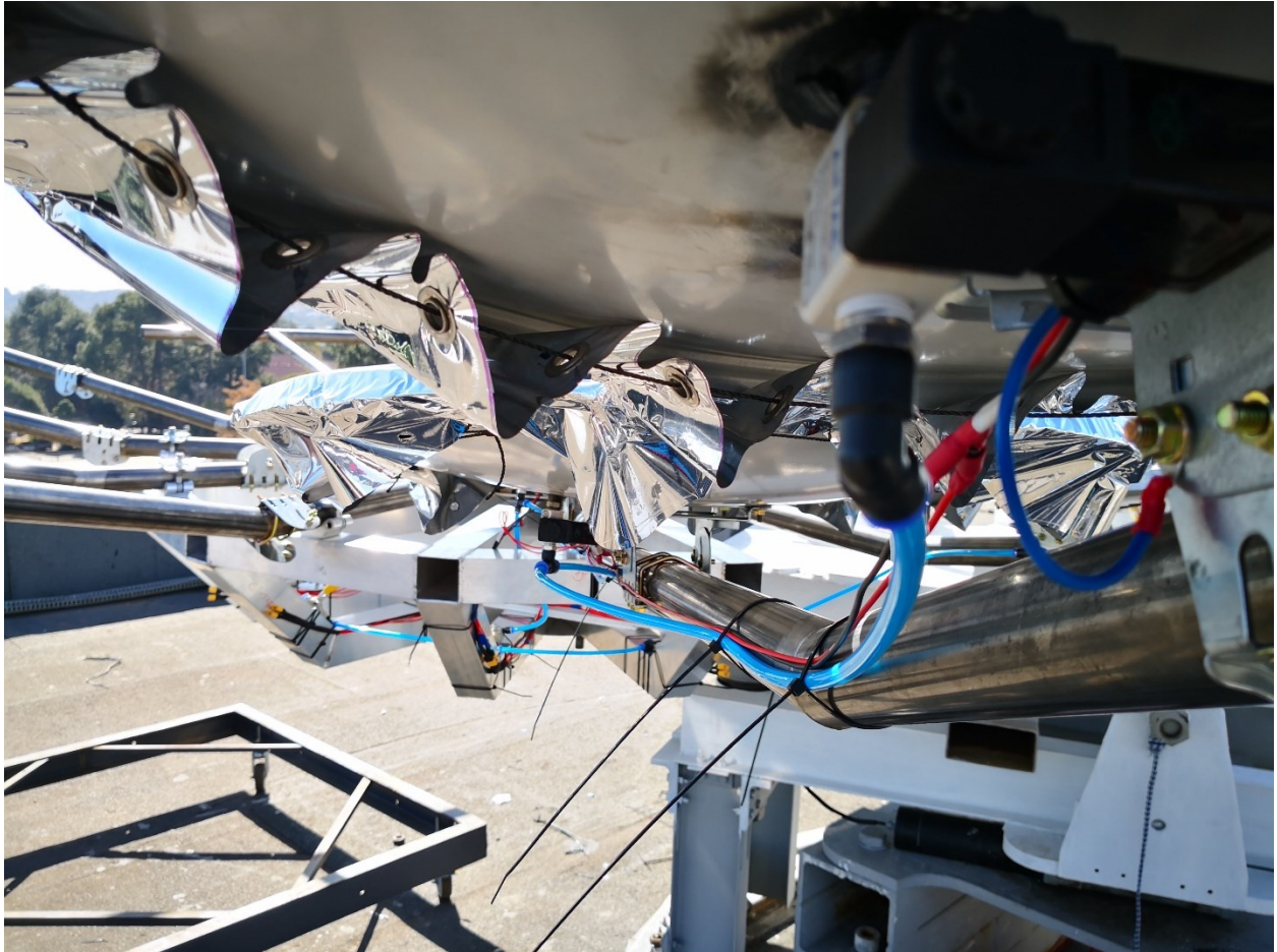
Figure B.1: Pneumatic line with solenoid and wiring used to control individual facet vacuum pressures. Pneumatic and electrical ring-line visible on the support frame.
