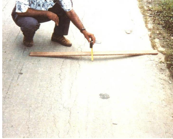
Figure 2-13: Wide subgrade rutting (SANRAL, 2014)
