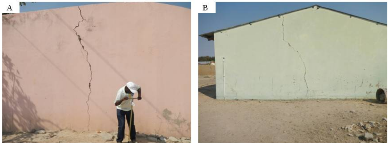
Figure 32: Cracking houses surveyed showing cracks with no particular orientation and in A, the cracks widen towards the top.
