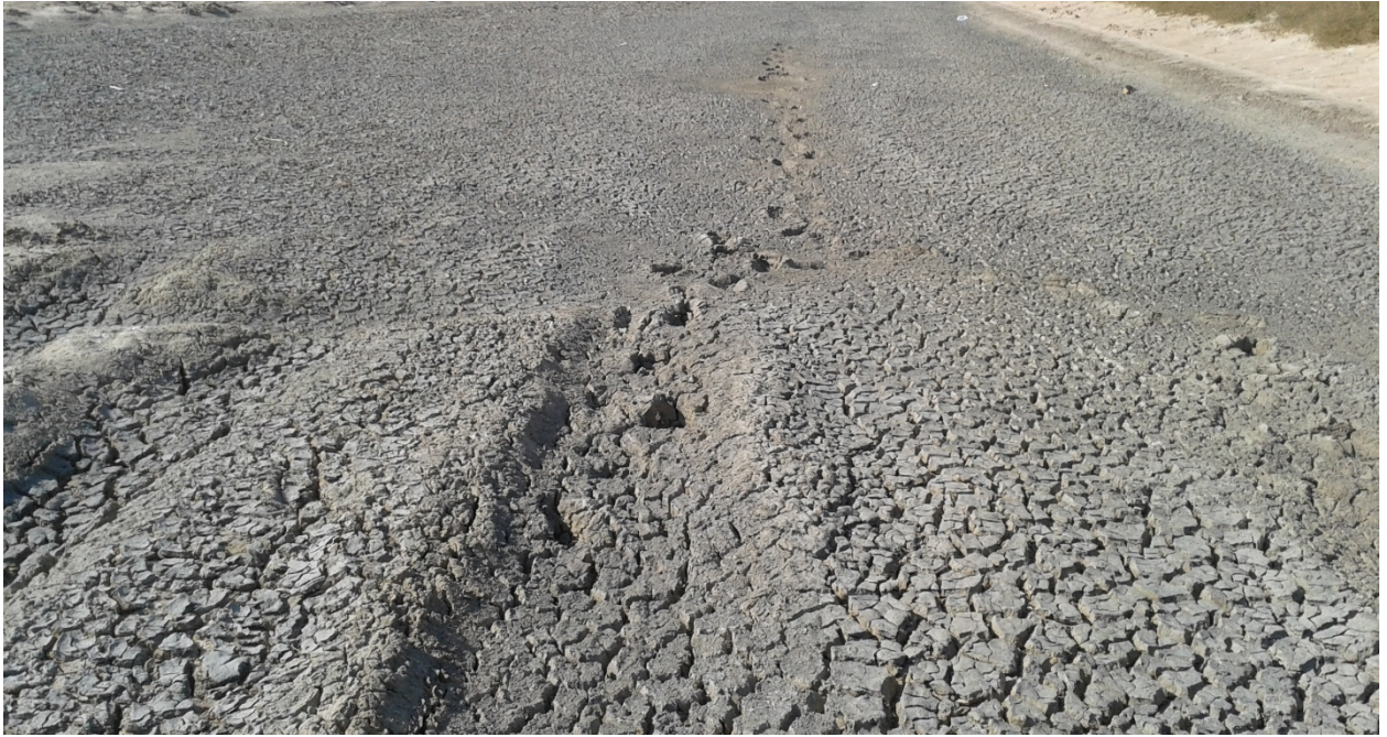
Figure 28: The desiccation cracks found in Land Facet 1.
