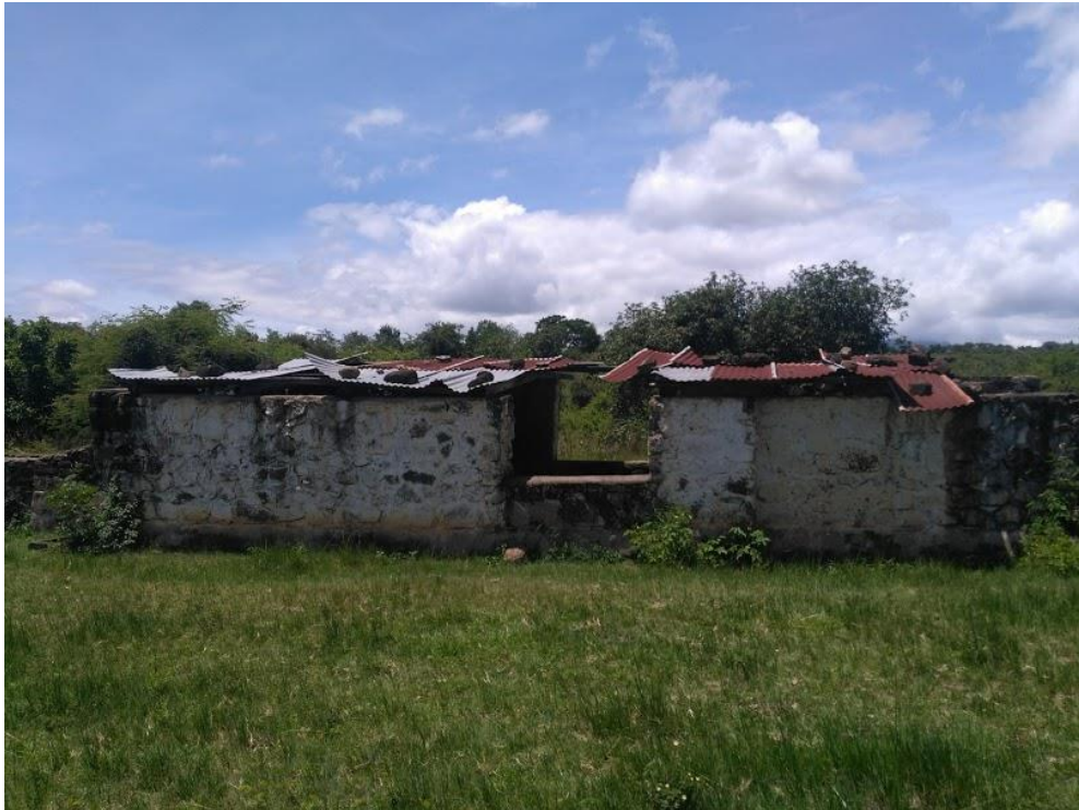
Figure 3.7: Communal dip tank in disrepair in Honde Valley, Zimbabwe (Photograph by ET Nyahangare)
