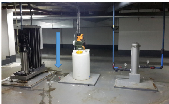
Fig. 2 Series of filters and reverse osmosis pump (right to left). Note the leak noted around the reverse osmosis pump (blue arrow)
