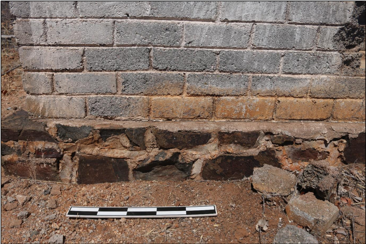
Figure 5.37: Stone foundation of Building 1 with grey brick wall on top. Area B.
