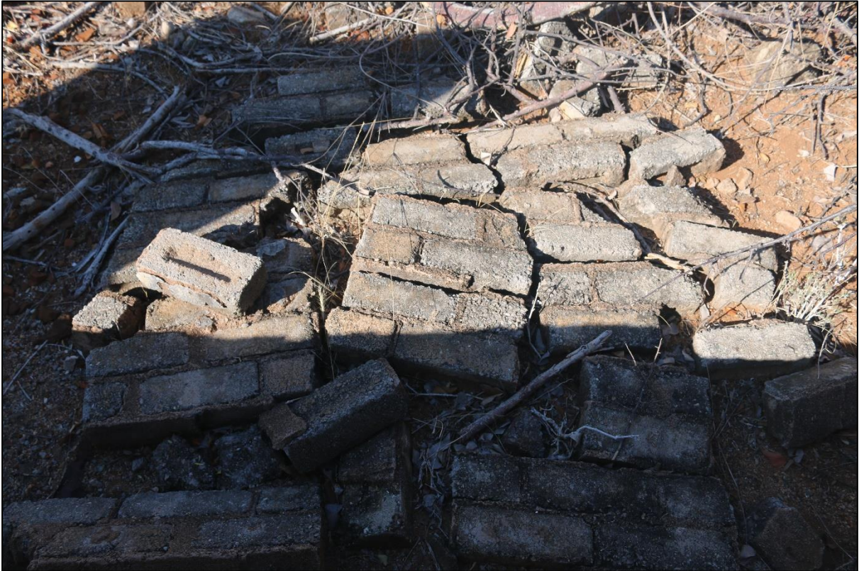
Figure 5.43: Broken down wall located outside of Building 1.
