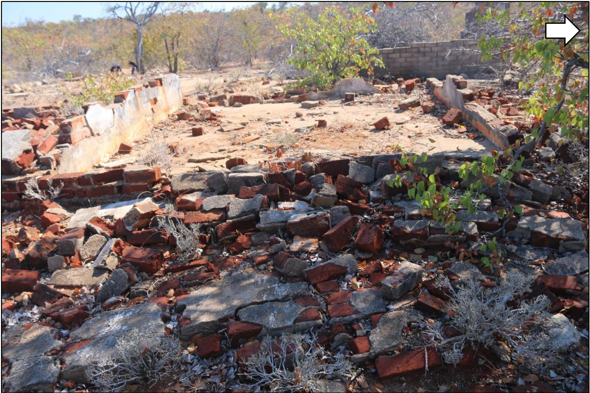
Figure 5.68: Collapsed wall (room 2.2) of Building 2.
