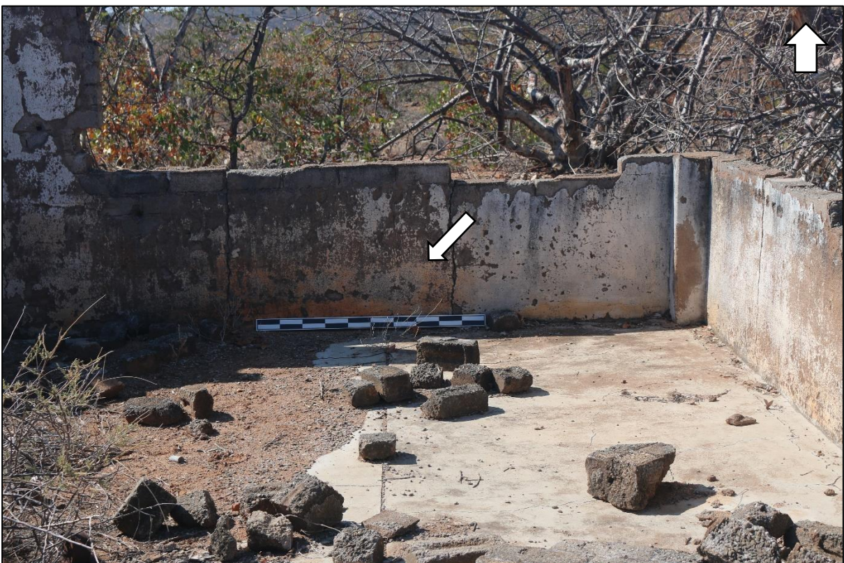
Figure 5.41: Eastern room (1.2) and inside wall, including the plaster on the wall, yellow/orange tinge from sun damage, is visible. Area B.
